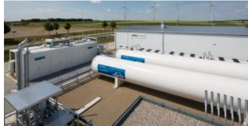
Wind to Gas to Power Energy Park in Mainz. In operation since 2015.
